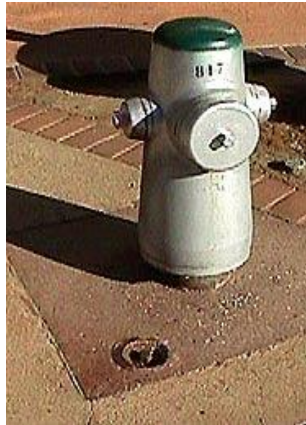
This hydrant has the valve stem in the sidewalk area.
